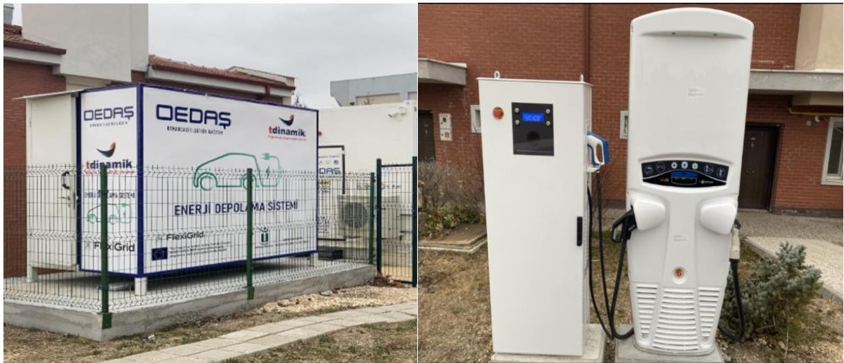
Figure 1 Battery Storage System (left), V2G and DC fast charging stations
